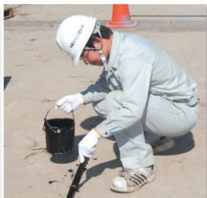
wire rope greasing
