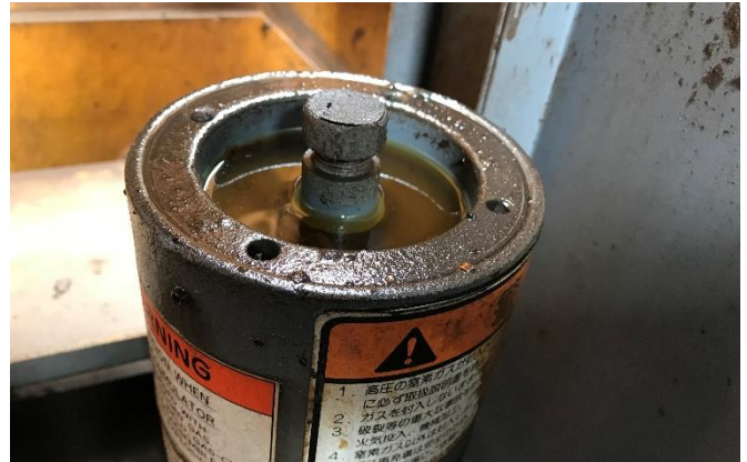
Oil leaking caused by bladder damage
